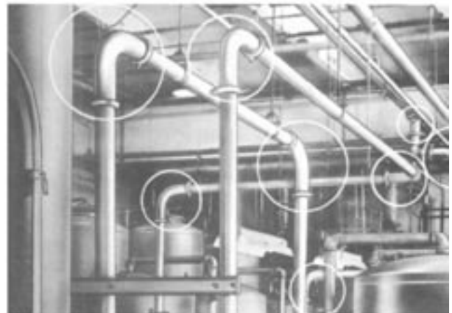
A large dry-cleaning plant uses Flexmaster joints to connect piping at elbow junctures.
